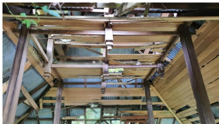
Figure 2: The very dilapidated state of Kampung Pelangai heritage masjid. (Source: Author, 2021)
