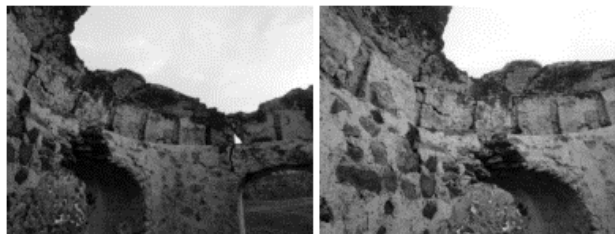
Figure 7. One of the structure damaged wells
