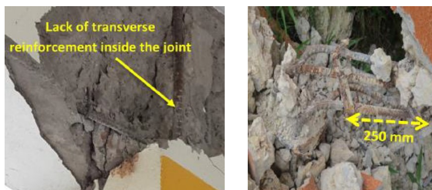
Figure 1: Damaged columns due to inadequate/poor detailing of confinements Source: (Alih & Vafaei, 2019)
