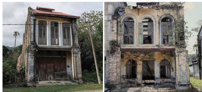
Figures 1 and 2: Dilapidated buildings in Papan, Perak Source: TSL Media Group, 2021
