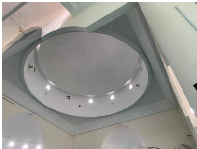
Figure 2. Defect: water leaking Source: Authors (2024)
