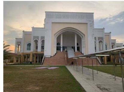
Figure 3. Defect: peeling of paint (external wall) Source: Authors (2024)
