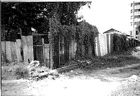
Photo C2.a: Zinc perimeter fencing – visual blight.
