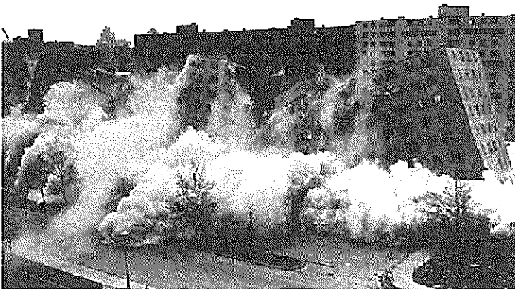
Figure 2: The Pruitt-Igoe housing development had to be torn down, at a loss of US$300 million, after it was declared unfit to be lived in. (Source: Newman, 1996, pg. 12)
