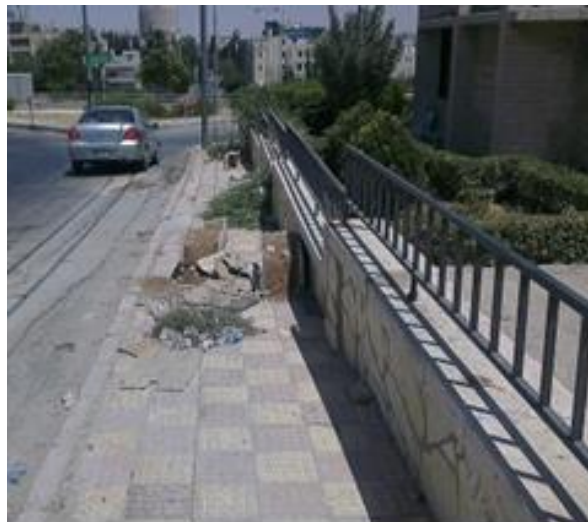
Figure 1: Example of poorly maintained sidewalk in Amman Source: Jafra News, 2015
