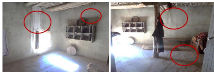
Figure 3 Cracks on the interior wall Source: Author
