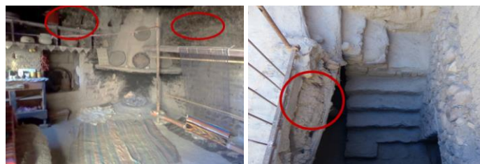
Figure 4 Poor condition of the common room walls (left) and stairs (right) Source: Author
