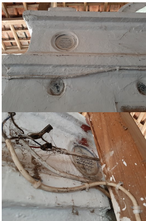
Figure 2: Ancient ceramics become a unique decoration in the grave complex of Sunan Gunungjati which is indicated to be damaged
