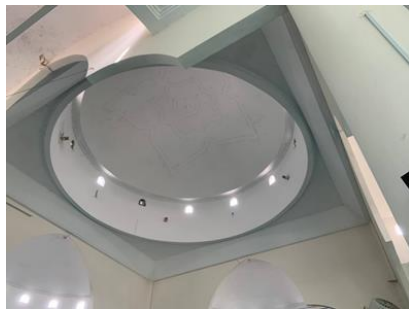
Figure 2. Defect: water leaking Source: Authors (2024)
