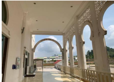
Figure 4. Defect: stagnant water Source: Authors (2024)
