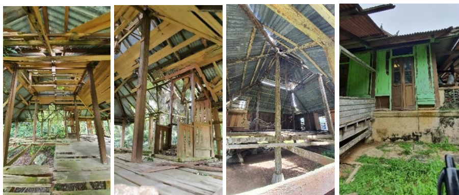
Figure 2: The deteriorating condition of timber structural elements.
